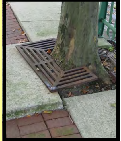
A TRIP AND FALL ACCIDENT WAITING TO HAPPEN...
