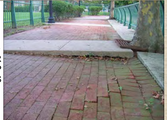
▶ MAJOR TRIP HAZARDS
