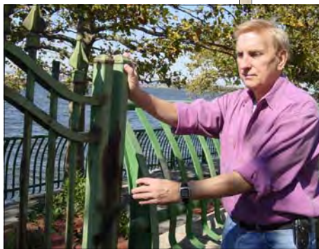
Vern Carlson inspects rusted, non-working gate on the Newark Bay Walkway.
