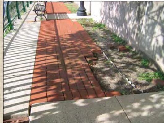
◀ UNSIGHTLY MISSING BRICKS
